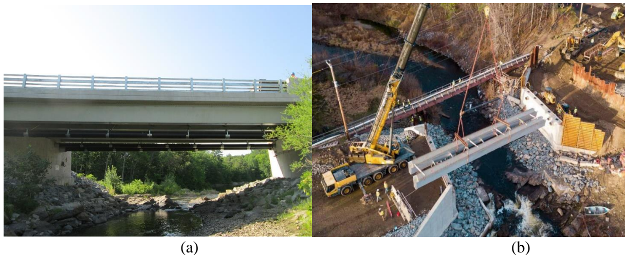
Figure 1.1: (a) HGMB Fully Constructed Looking Downstream, (b) During Construction with a Two-Girder System Being Set by an Individual Crane
