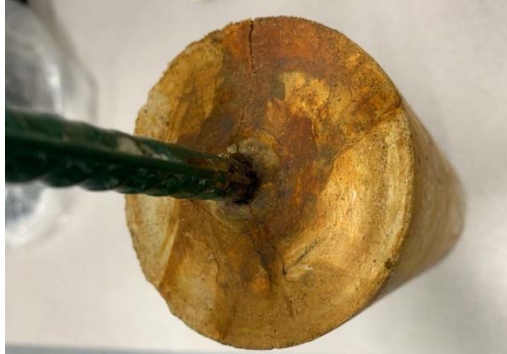
Figure 3: Close-up of damaged RC cylinder.
