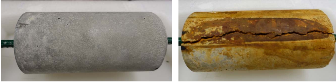
Fig. 1: Intact (0% corrosion) RC cylinder (left) and fully corroded (100% corrosion) RC cylinder (right)
