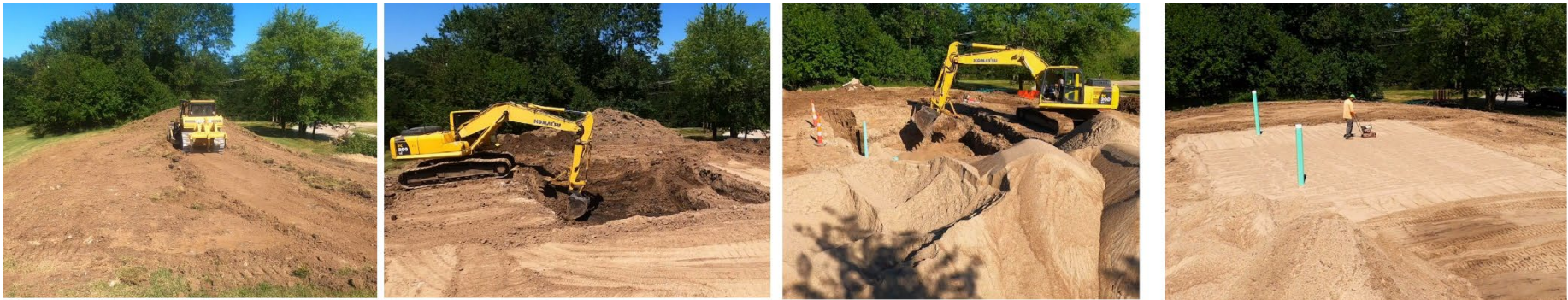
Figure 4. 30x25x8 ft Sand Pit construction sequence. Sand was compacted every foot intended to increase density and strength.
