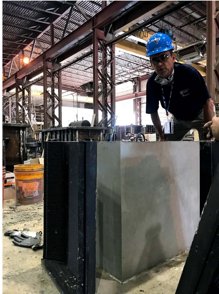
Figure 2 – PI Lopez-Anido inspecting 3D printed formwork after casting and demolding at the American Concrete Industries plant
