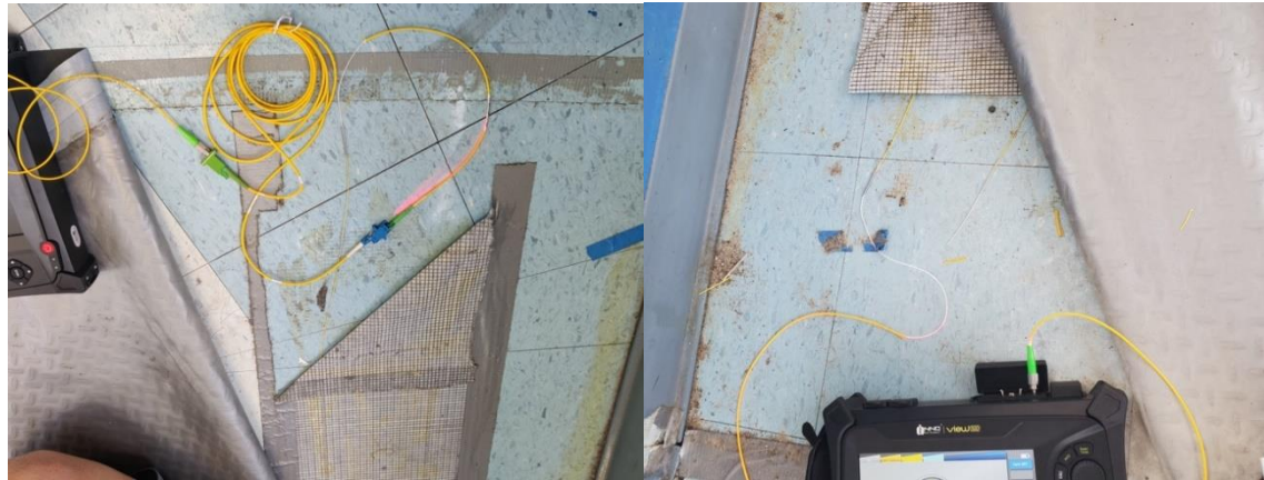
Figure 2 Photo of fiber connector on pedestrian bridge.
