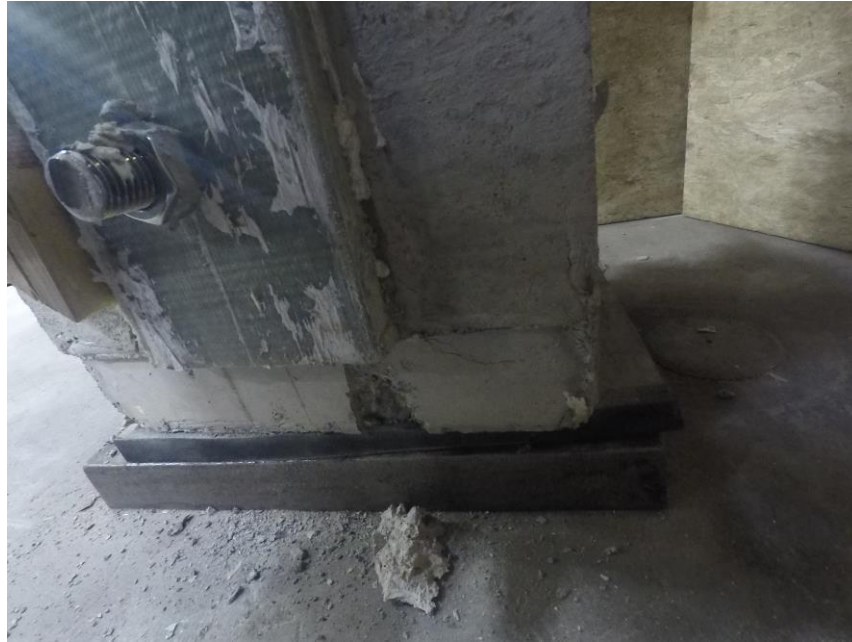
Figure 27: Specimen 3 – Minor Concrete Spalling
