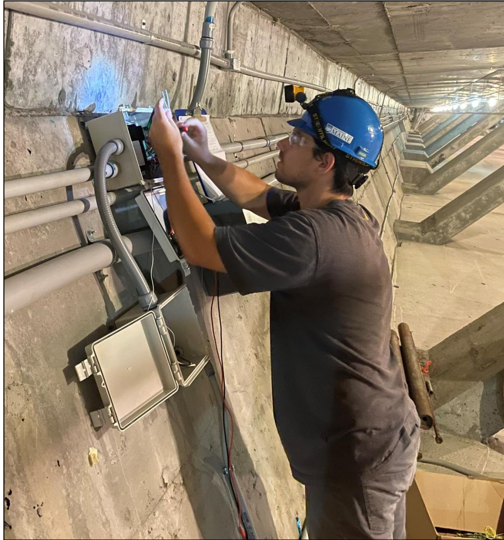
Figure 5. Undergraduate Jake Bear completing the instrumentation wiring to the wireless DAQ node at one of the stay anchorage locations.
