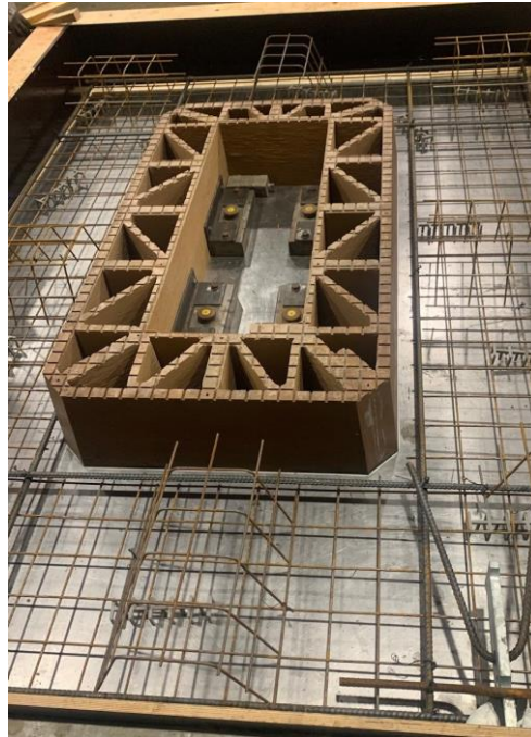
Figure 2 – 3D printed form of at the Unistress precast concrete plant in Pittsfield, MA.
