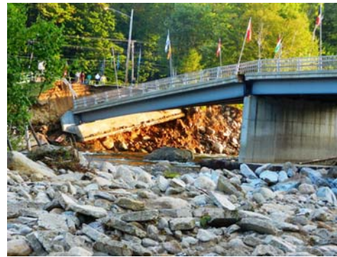
(b) Bridge collapse in New Hampshire from Tropical Storm Irene (HEB Engineers, 2011)
