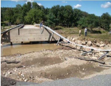
(a) Bridge collapse in Vermont from Tropical Storm Irene (Hewitt, 2016)
