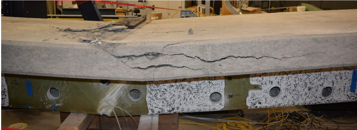
Figure 4-13: Image UTC-4 of Failure Location and Damage
