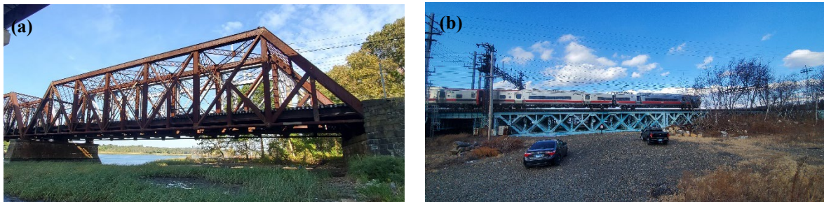
Figure 5: (a) Devon bridge span 7 from the south bridge, (b) Cos Cob bridge span 3 from north bridge
