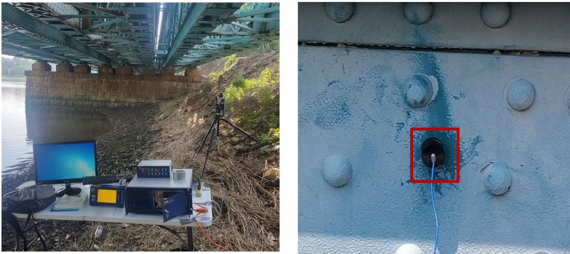
Figure 18: LDV setup to record vertical response, Laser beam pointed to node at the intersection of bottom chord and vertical members (1), Accelerometer attached to bottom chord of Cos Cob Bridge for reference (2)
